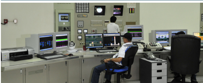
Pagbilao Control Room
