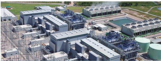
Ratchaburi Power Plant
